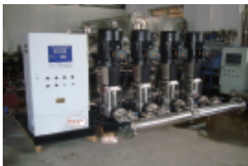
Constant pressure water supply
